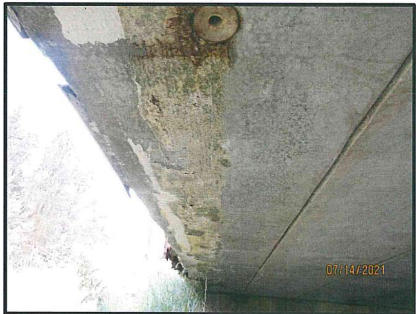
41-249-268 Deterioration of South Exterior Beam
